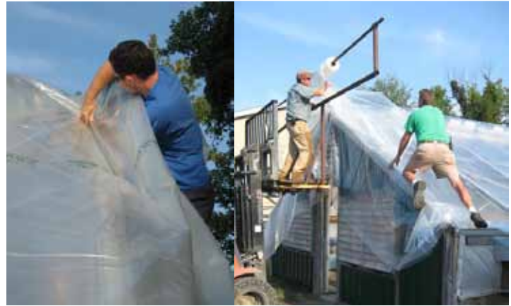
Fig. 3. Replacing plastic on bubble system greenhouse; Canadian expert installing splines (left); UVM and Claussen employees rolling out plastic (right).
